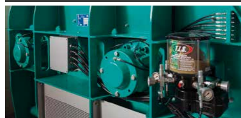
Automatic lubrication system equipped with 4 programmable and independent pumps
